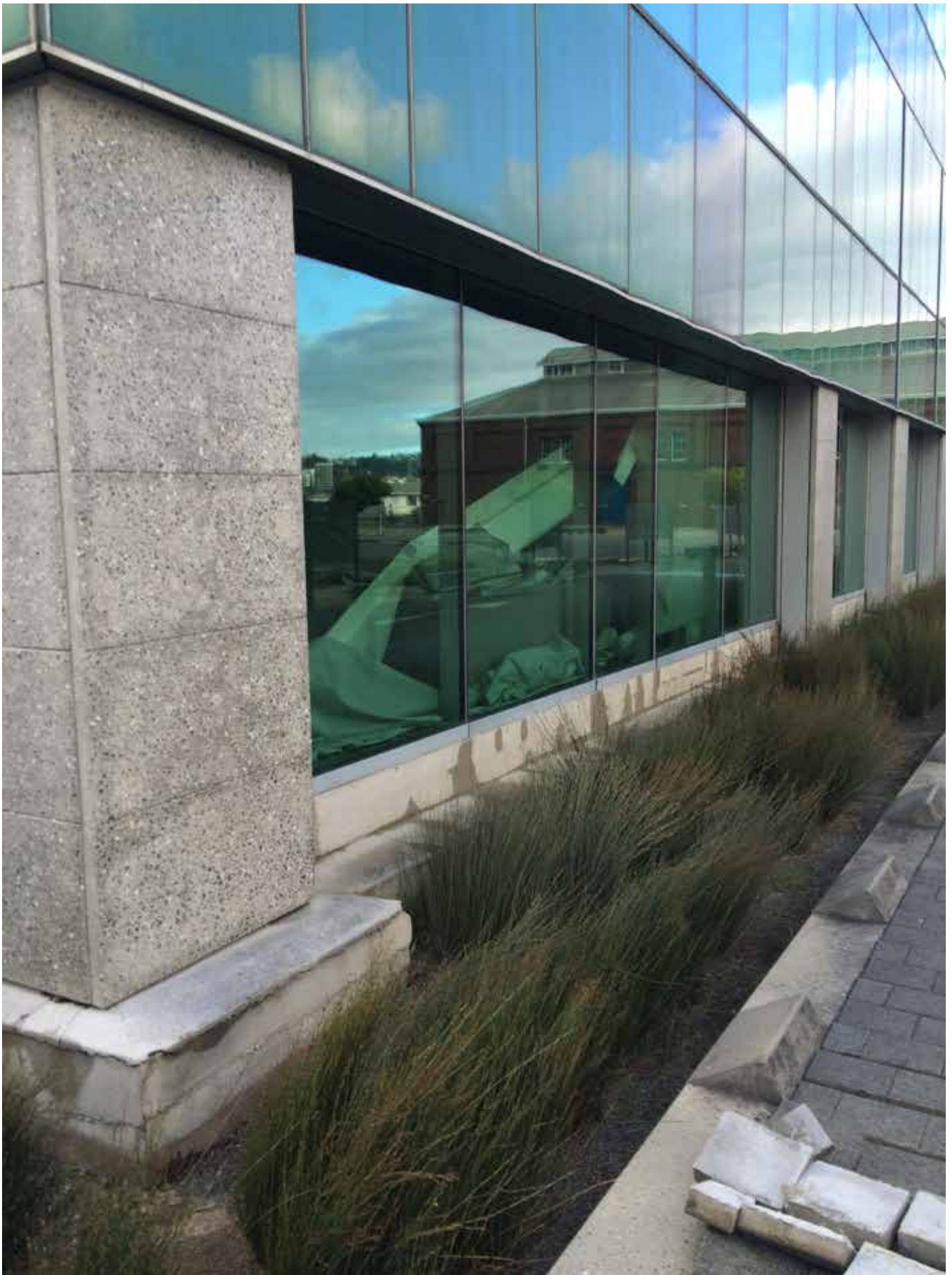
Damage to Statistics House following the 2016 Kaikōura earthquake. Photo: Statistics New Zealand.
