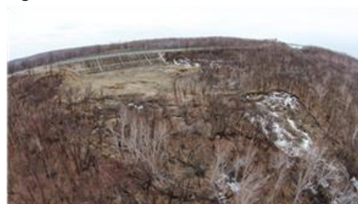
Figure 14. View of the K177+550 landslide
