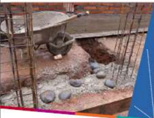
Image 1: Tie-column reinforced cages extending from foundations of a new building; these are a key feature of 'confined masonry' construction. Source: Stacy, Astiza and Yedlin, 2010 1 .
