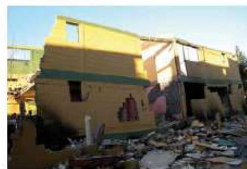
Image 2: A building with a collapsed ground floor as a result of the February 2010 earthquake in Chile. Source: Stacy, Astiza and Yedlin, 2010 14 .
