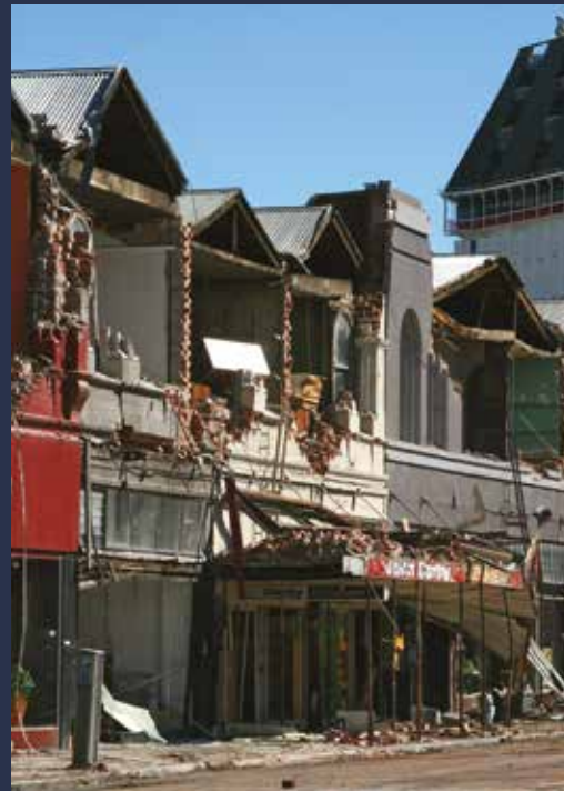
▲ Clockwise beginning Top, left: Rockfall following the Christchurch earthquake. Photo: GNS Science; Damage in Greymouth after ex- Tropical Cyclone Ita. Photo: NIWA; Building damage caused by the Christchurch earthquake. Photo: GNS Science; Damaged irrigators following Canterbury wind storm. Photo: NIWA.
