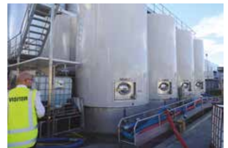
▲ Top: University of Auckland PhD student, Mohsen Yazdanian inspecting damaged wine tanks in the Marlborough following the 2016 Kaikōura earthquake. Photo: Dmytro Dizhur.
