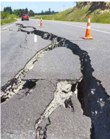
▲ Road damage near Clarence caused by the 2016 Kaikōura earthquake. Photo: Julian Thomson, GNS Science.
